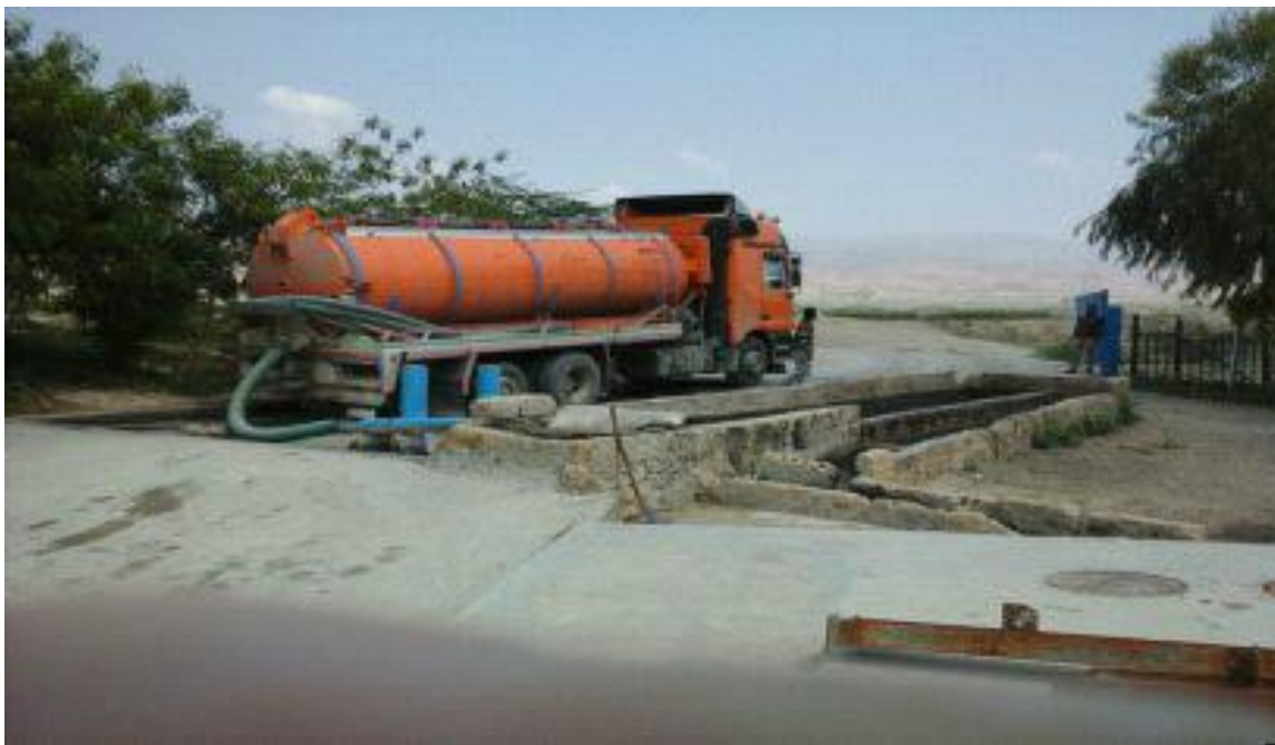
Figure (1.3-C) Septic Tank emptying to the WWTP Headworks
